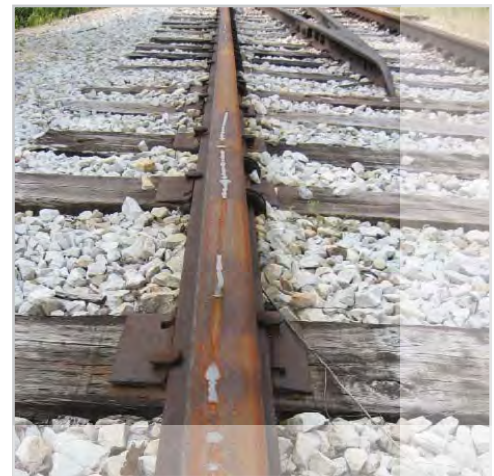
FALL CREEK TRACK CONDITION
